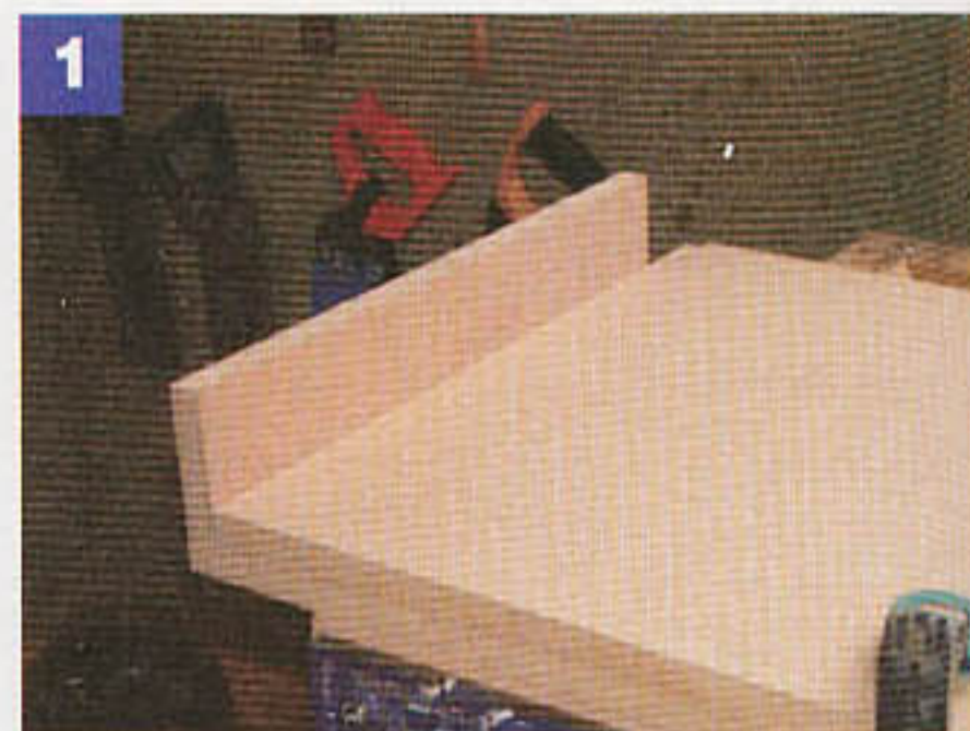
1 Use a piece of scrap 18mm thick board as a spacer for setting up the biscuit joint
